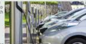
Electric Vehicle Charging Point
